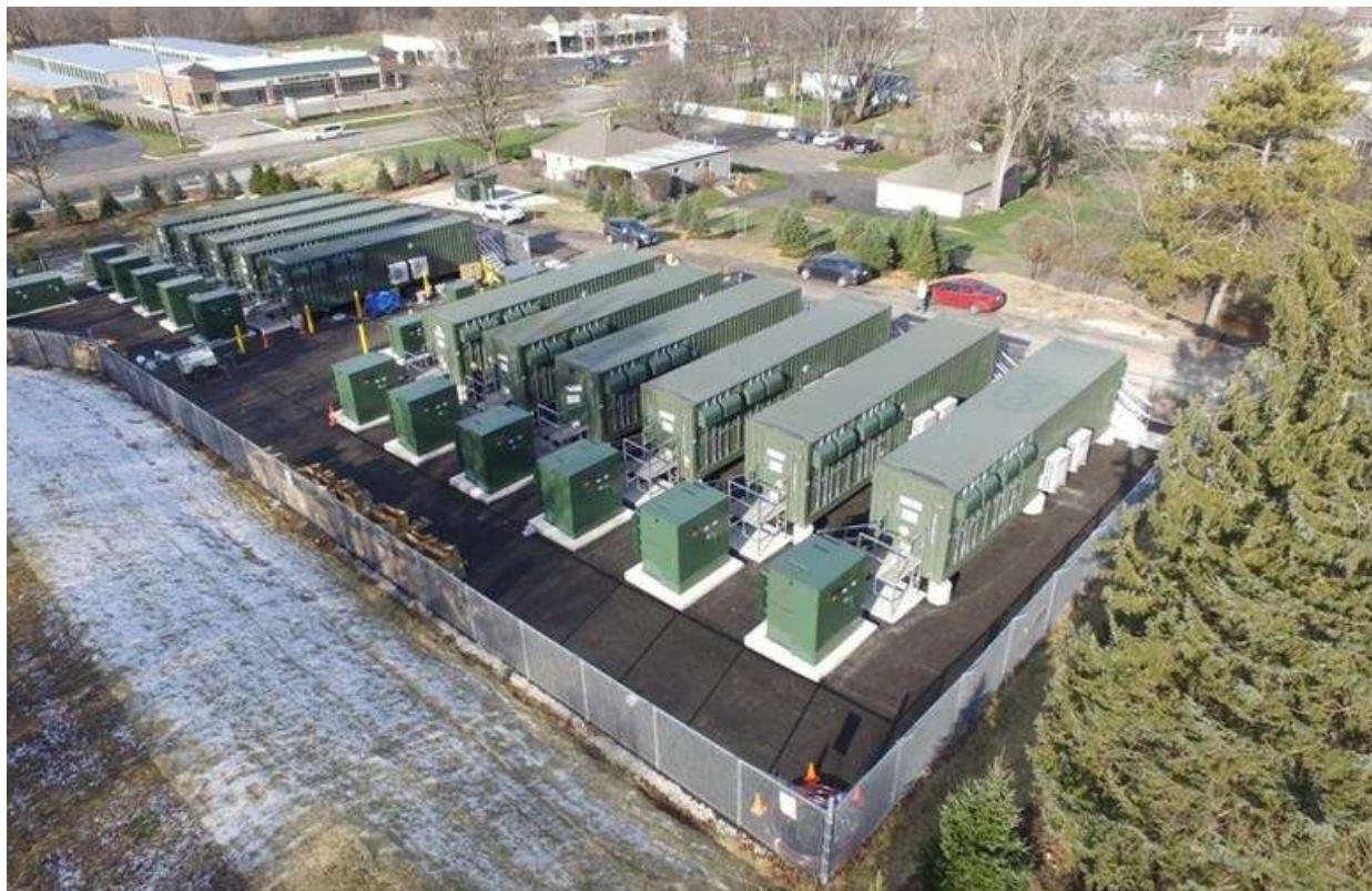
EDF 20 MW BESS (BYD America cells) em Illinois / USA
