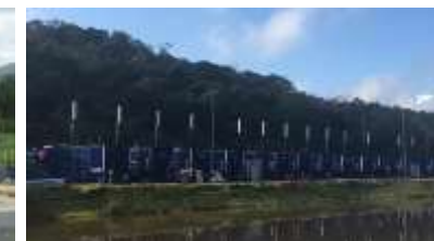
Gas Natural – 20 MW Sabesp, São Paulo
